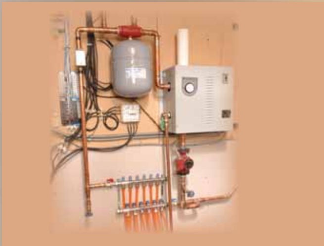
Electric boiler system with oil or gas fired boiler backup
