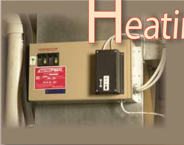
Electric plenum heater with oil or gas forced air backup
